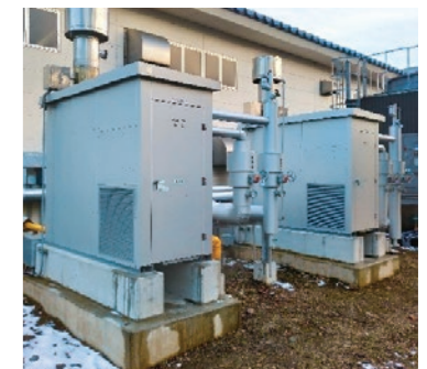
Hot water boiler
