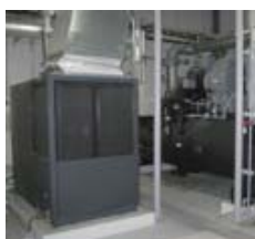
Inverter turbo refrigeration machinery
