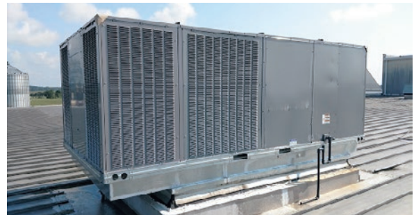
High-efficiency air conditioning unit
