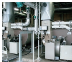
Vacuum hot water boilers
