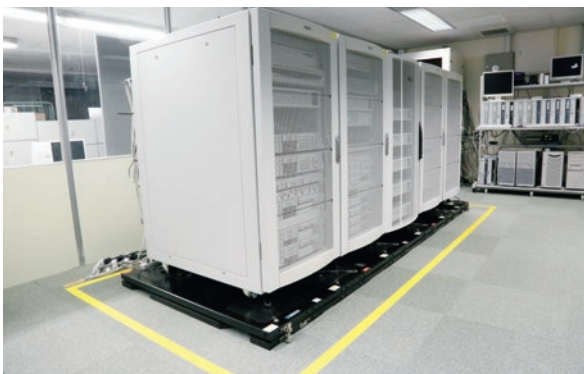
Servers that kept functioning during the Kumamoto Earthquakes thanks to seismic isolation systems
