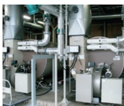
Vacuum hot water boilers
