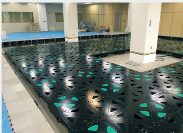
Server room equipped with custom-designed seismic isolation devices from THK
