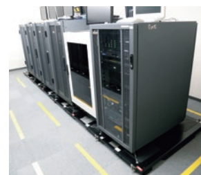
Servers with seismic isolation devices
