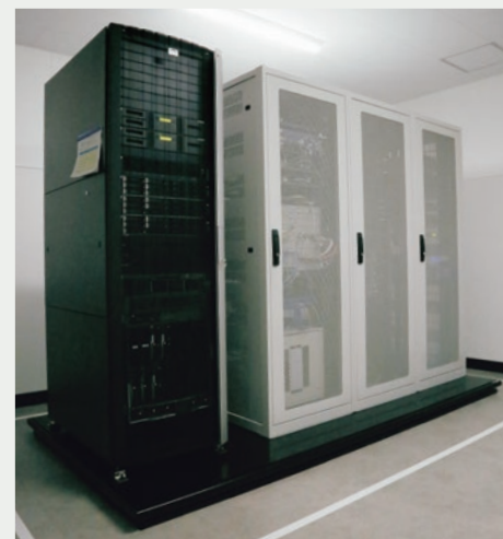
Servers in our new emergency shelter, safeguarded by seismic isolation
