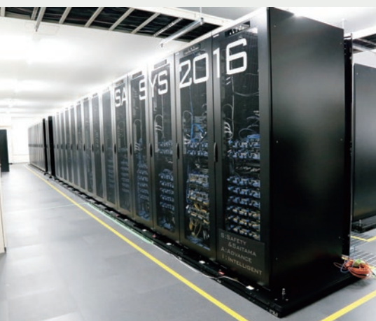
Seismic isolation devices safeguarding our servers
