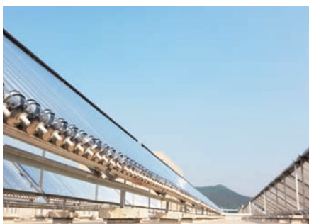
Solar power is collected to heat the plant's water. Some of the water is used for the plant's showers and heating system.
