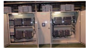
Inverter control panels.
