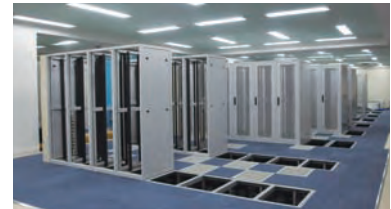
The entire transmission room floor is protected by seismic isolation devices.
