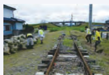
Railroad tracks damaged in the tsunami.
