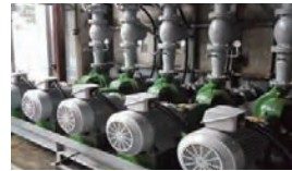
Coolant pump motors.
