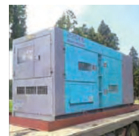
Electric power generator used at THK NIIGATA.
