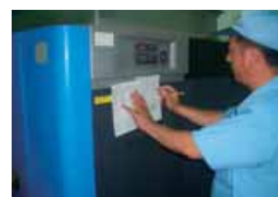
Periodic compressor inspection
