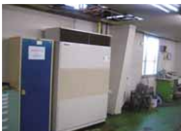
An air-cooled air conditioner
