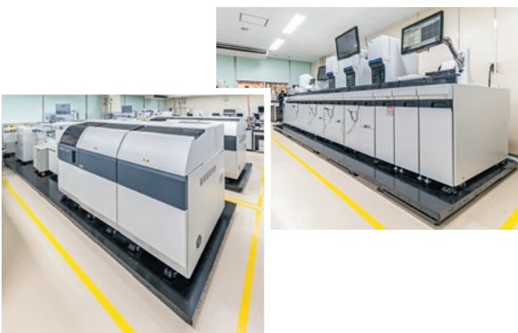
Blood analyzers (top right) and biochemistry auto analyzers (bottom left) installed with seismic isolation systems
